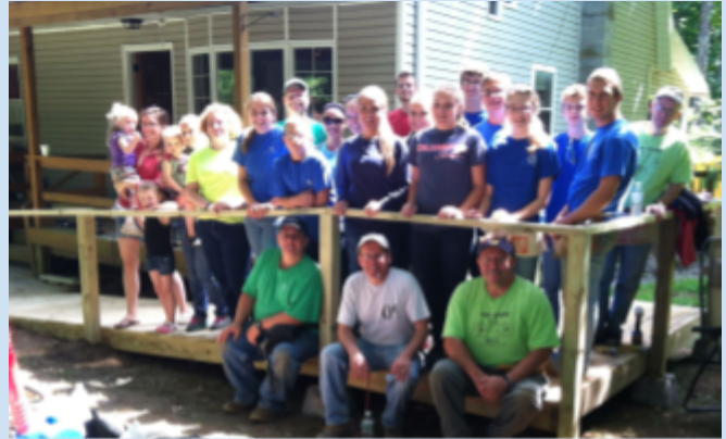
St. Mark's handy teens work together to build wheelchair ramps for those in need each summer.
